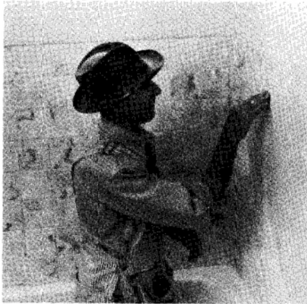
Art Hunter places tile on the bathroom wall in the old office building.
